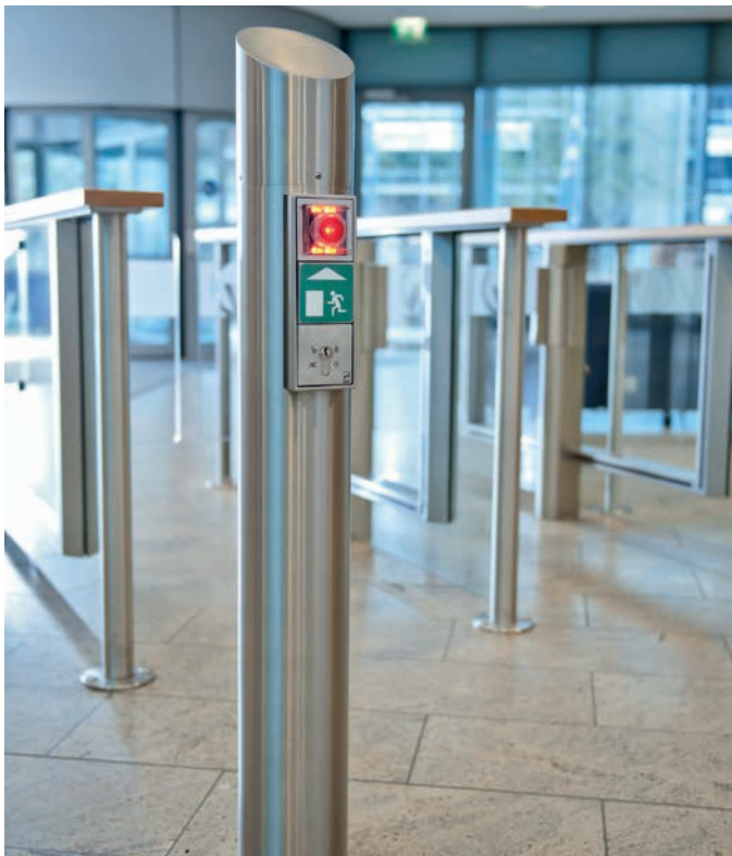
Card reader post with escape route terminal
